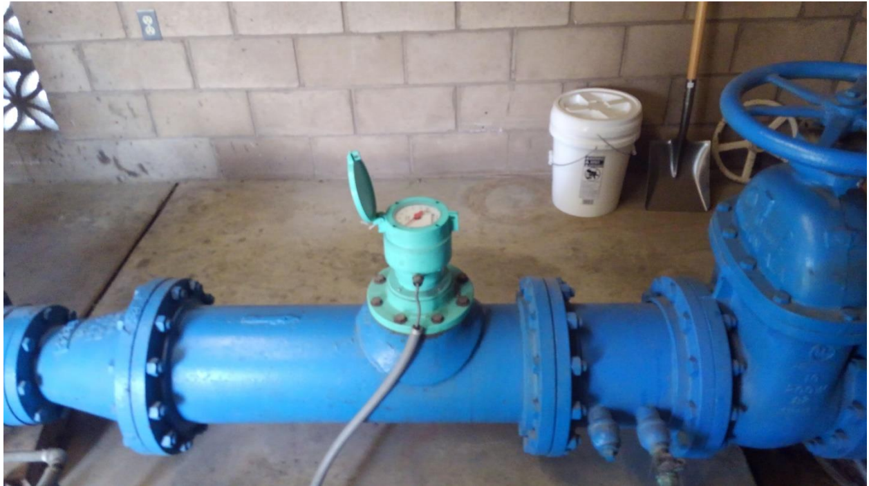
Figure 3d. Sample current propeller flow meters, to be retrofitted with magnetic flow meters
