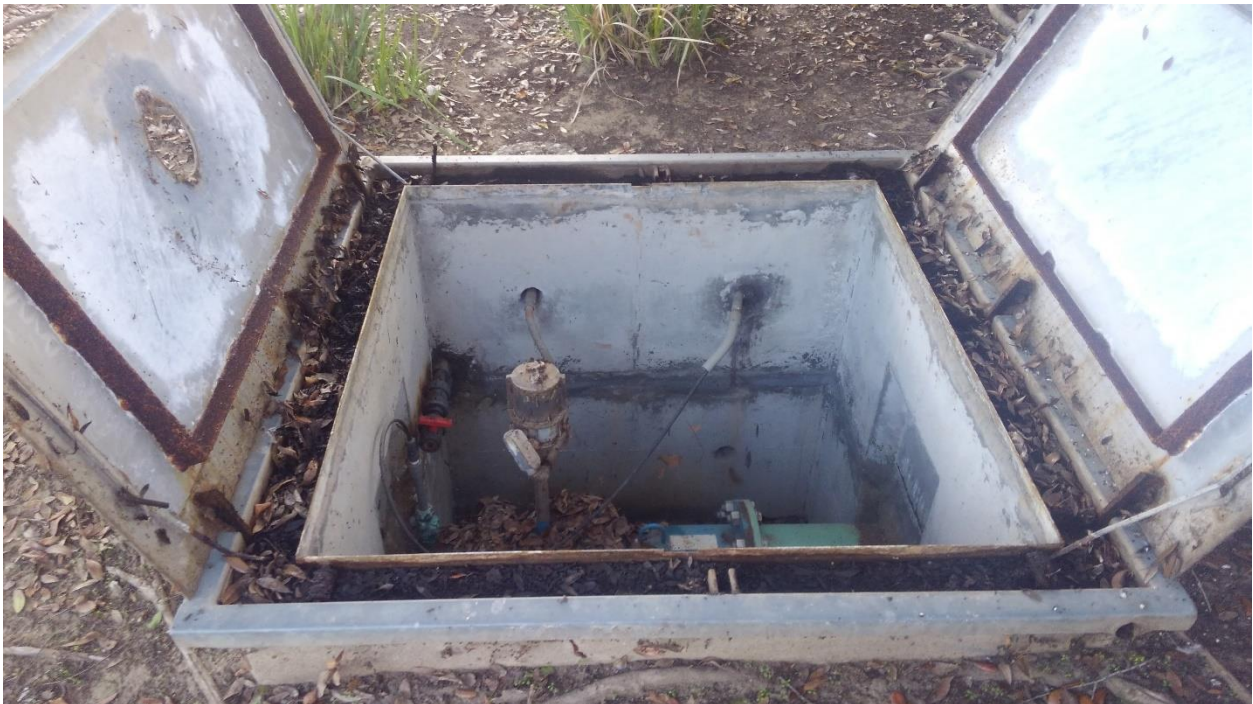
Figure 3b. Sample well-site facility 2
