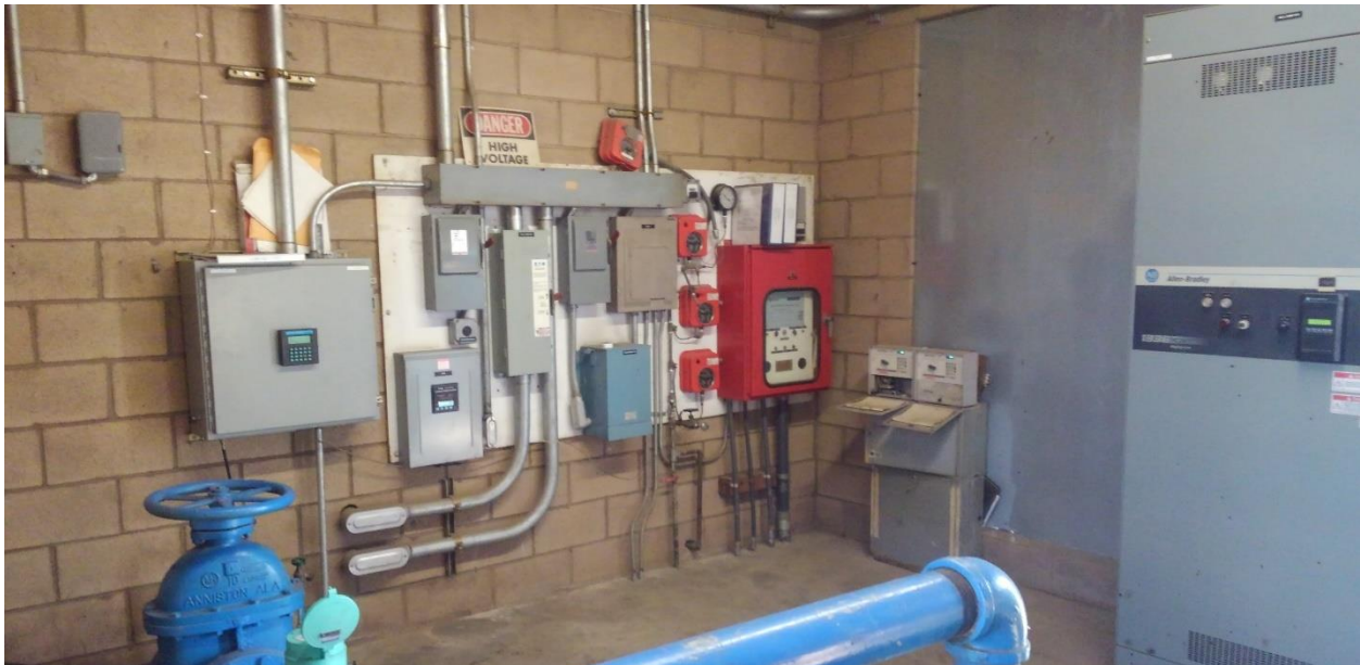
Figure 3c. Sample well-site facility interior, site of PLC installation
